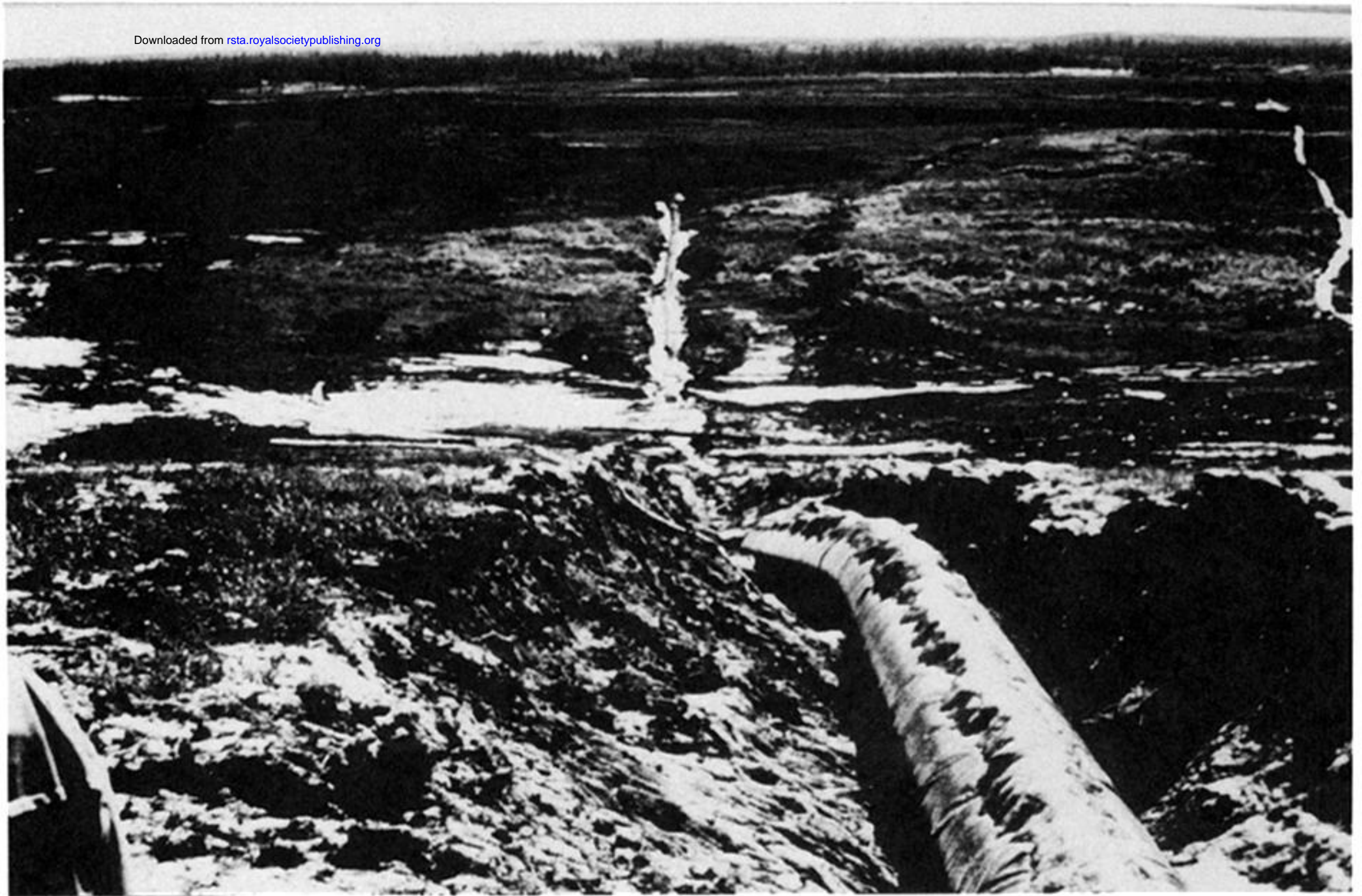
Figure 2. Large pipeline exposed by erosion following freezing, heaving and thawing of near surface layers above permafrost (Siberia). Photograph by E. D. Ershov.
